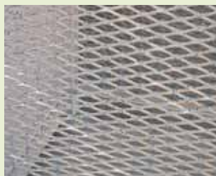
▼ Deteriorated polyester coating after 6 years.
